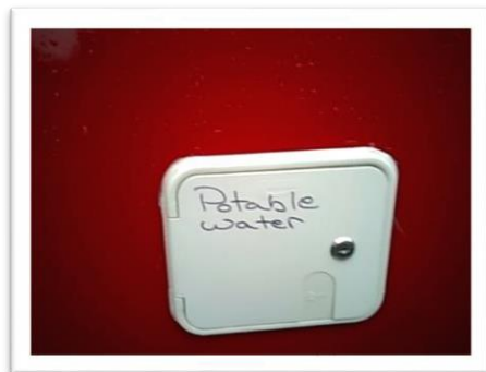
Potable Water Inlet
