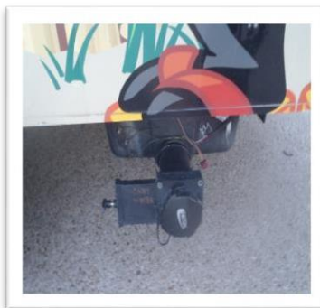
Liquid Waste Connection
